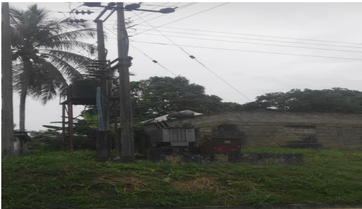
Figure 4.1: Shows the 33KVA electrical transformer donated by Community-Based Organization in Isinkwo community, Onicha LGA, Ebonyi State
