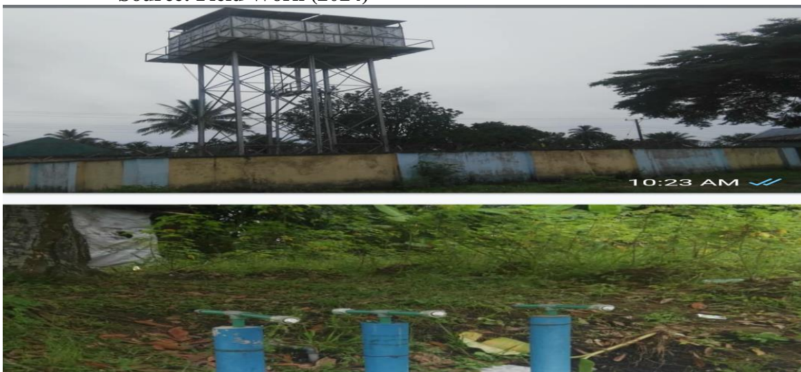
Figure 4.4: Shows a Solar inverter water project donated by Community-Based Organization in Onicha-Igboeze community.
