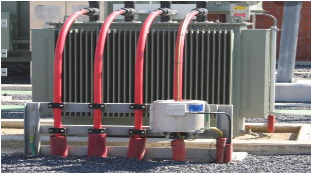
Figure 4.2: Shows a 33KVA electrical transformer donated by Community-Based Organization in Isu Community, Onicha LGA.
